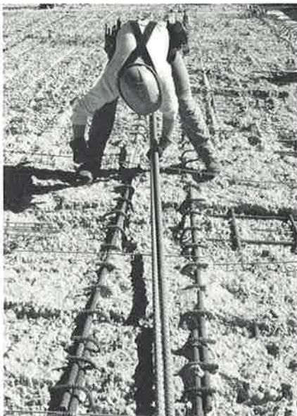
Installation of new rebar became necessary after concrete deterioration led to exposure and corrosion of reinforcing steel in this concrete structure.
