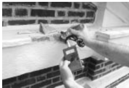
Determining the moisture content of subsurface masonry is a frequently used investigative method that can help identify the integrity of back-up materials.
