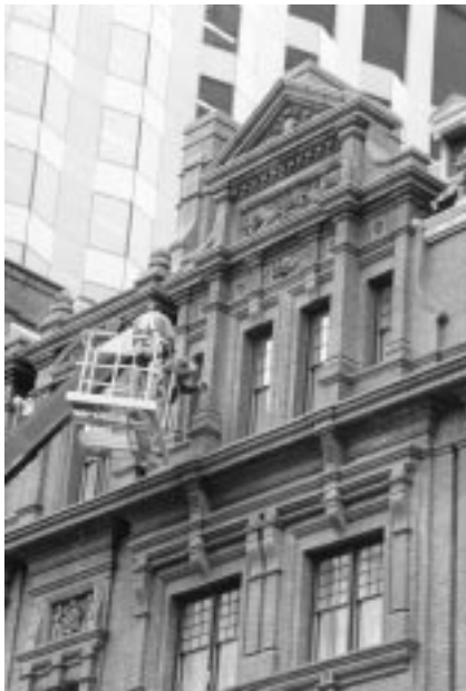
Paul C. Lanteri, AIA investigates masonry deterioration at the turn-of-the-century Goodwin Hotel in Hartford, CT.
