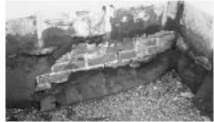
This repair effort used roofing cement to seal over a leaking brick parapet wall — a solution that instead trapped moisture within and caused further deterioration.
