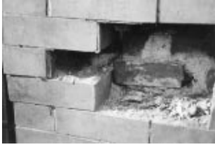
Behind the brick face of this historic structure, a probe reveals interior masonry that has disintegrated to powder. Note also the dramatic brick displacement and lack of a proper seal at the mortar joints, which can lead to moisture infiltration and further damage.
