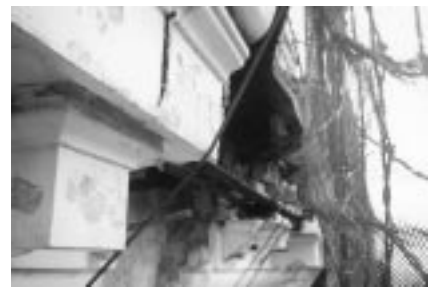
As an emergency measure, netting was installed on this severely deteriorated, 80-year-old cornice to prevent loose materials from falling.
