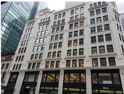
▲ Open Society Foundations Headquarters, New York, NY, Facade Repairs, Including Replacement of Terra Cotta with Cast Stone.
