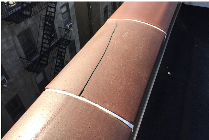
Cracked terra cotta coping stone poses a potential hazard.
