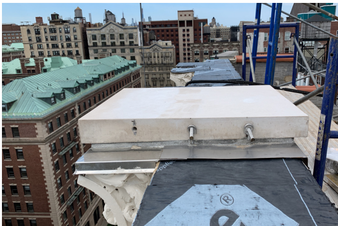
Parapet reconstruction incorporating waterproofing membrane, flashings, precast coping stones, and steel anchors.
