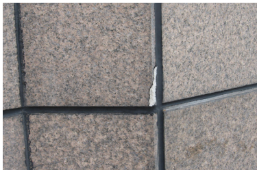
Repair "SWARMP" conditions from Cycle 6 before they become "Unsafe" in Cycle 7.
