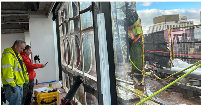
A Other cities may follow NYC's lead in requiring whole-building air leakage testing, a major change from the earlier code.
