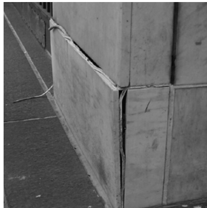
Sealant and anchorage failure
