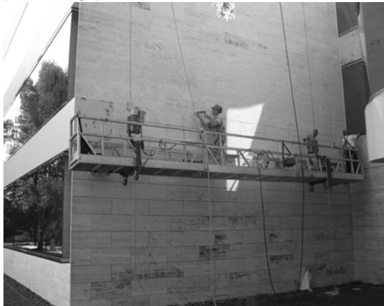
▲ Periodic sealant replacement should be part of a comprehensive maintenance program.
