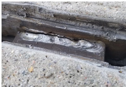
▲ Failed connection due to fatigue stress.
