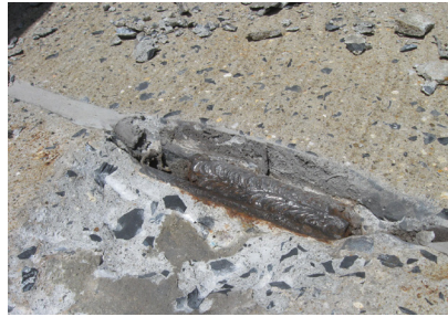
▲ Edge spall due to the heat of welding.
