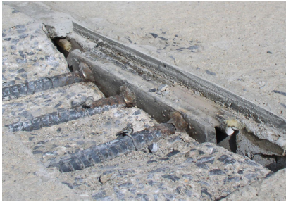
▲ Corrosion of dissimilar metals.
