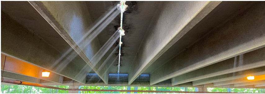
▲ Daylight shines through an open flange-to-flange joint during a connection repair project.
