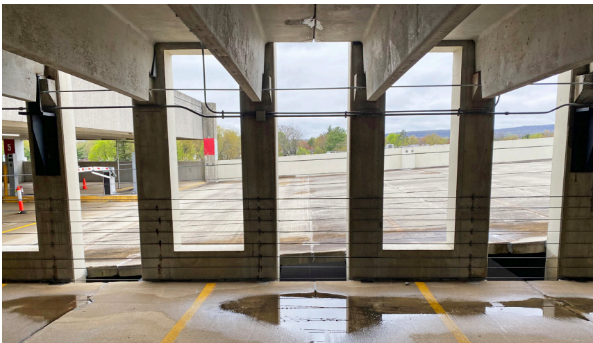
▲ Leaks and spalls might seem like minor nuisances, but they can signal serious structural distress.
