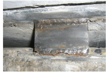
▲ Abrupt failure between tee and shear wall.
