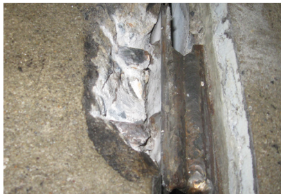
▲ Fractured rebar at flange connection.
