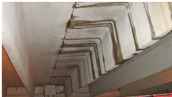
▲ Continuous leaks indicate failed sealant and, possibly, an unzipped joint.
