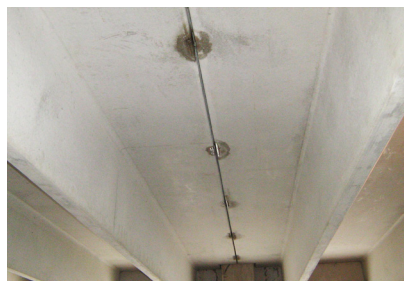
▲ Leaks at connections due to welding.
