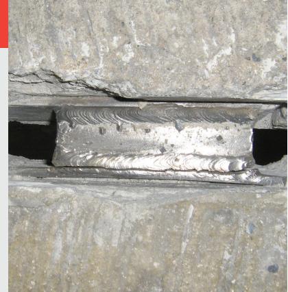
▲ Fractured flange connection caused by cyclical fatigue stress.
