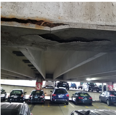
Regular inspection and repair prevents hazards and extends garage lifespan.
