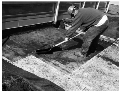
A Remediating a leak on a green roof involves removal of plants and overburden.
