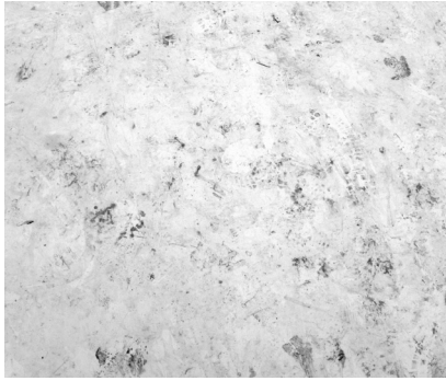
A Dirt and stains from foot traffic can compromise cool roof performance.
