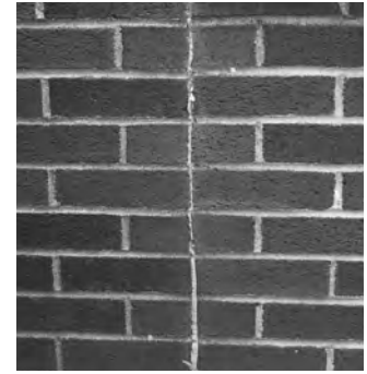
▲ Insufficient expansion joint width.
