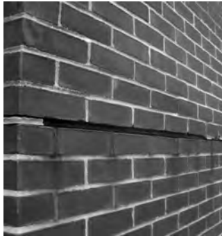
▲ Corrosion of steel shelf angle.
