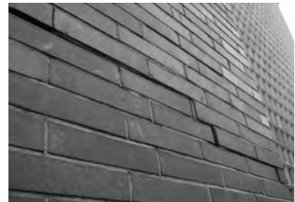
▲ Lateral displacement of brick veneer.
