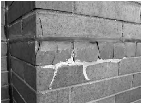
▲ Sealant alone cannot resolve masonry distress.
