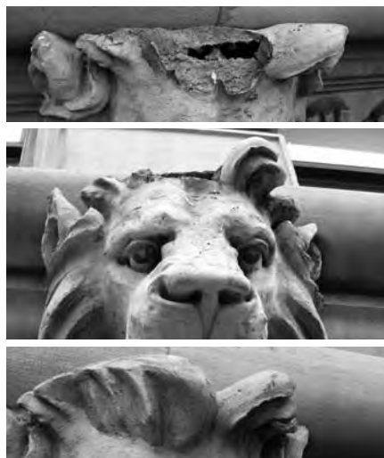
▲ Restoration of spalled terra cotta decorative element.
