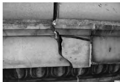
▲ Untreated deterioration can result in hazardous conditions.
