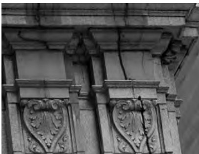
A Cracking at building corners.
