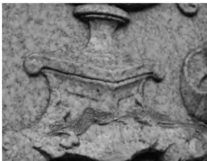
A Failed prior repair effort.
