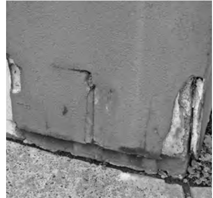
▲ Impact damage that is not repaired promptly provides a pathway for leaks.
