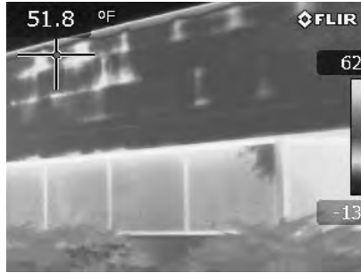
A This infrared thermographic scan reveals trapped moisture at insulation board joints.
