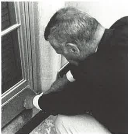
thorough investigation of the glazing system should determine causes of problems
