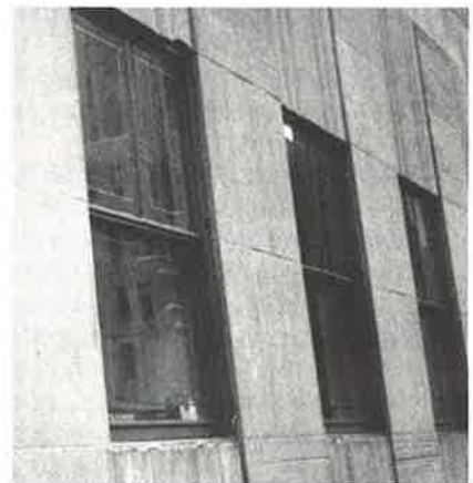
older single glazed windows are prime candidates for replacement
