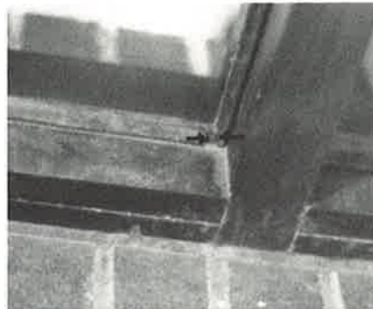
gap at corner of glazing gasket
