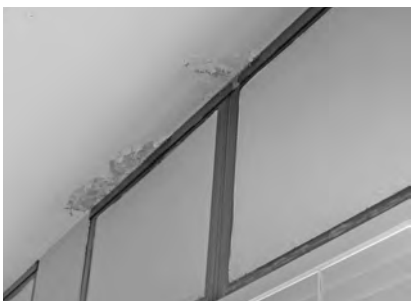
▲ Leaks and drafts.
