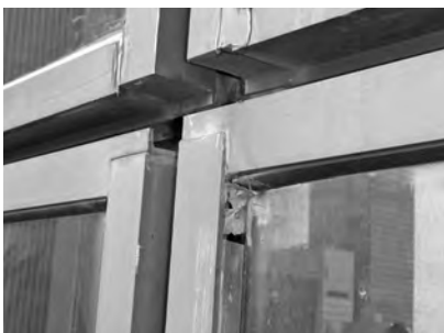
A Gaps at frame corners.
