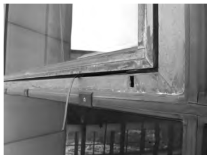
A Loose or missing weather stripping.
