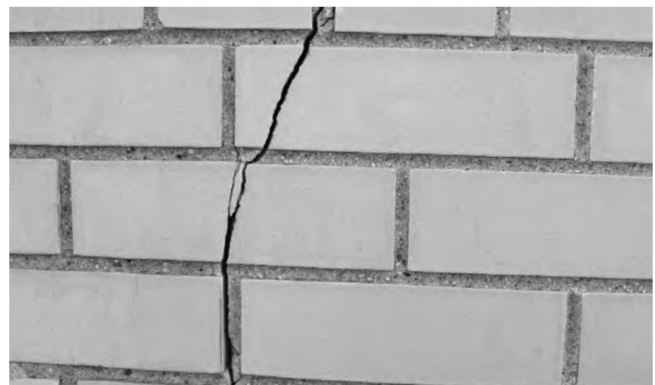
▲ Vertical crack in a glazed brick facade.
