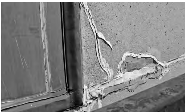
▲ Inappropriate crack repair using surface-applied sealant.
