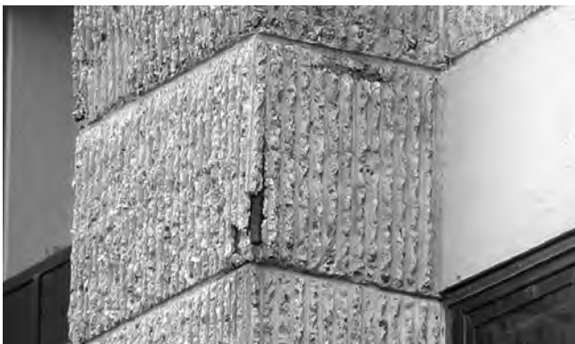
▲ Reinforcement corrosion and spalls in béton brut ("raw" concrete).
