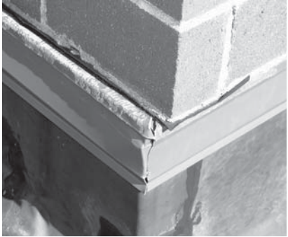
▲ Litigation support relating to roof design and installation errors at a primary school.
