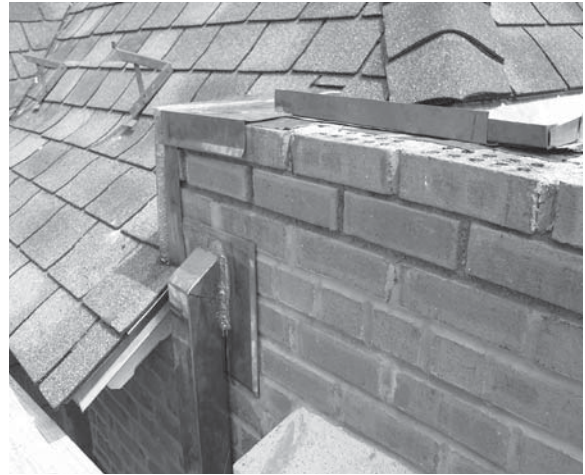
▲ Building intersections are susceptible to leaks. Paying extra attention to these vulnerable areas during construction is critical to failure prevention.
