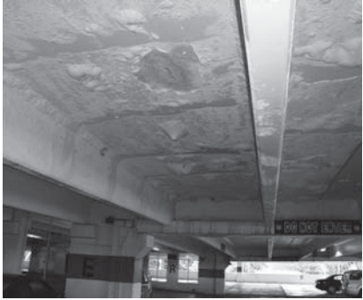
▲ Defect evaluation, remediation, and expert witness services for a hotel parking garage.
