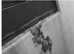
Exterior finish damage.
