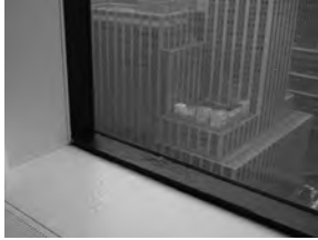
Water pooling at sill.
