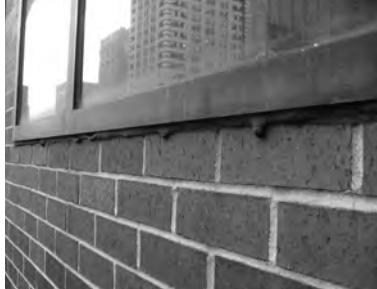
Sealant failure at window exterior.
