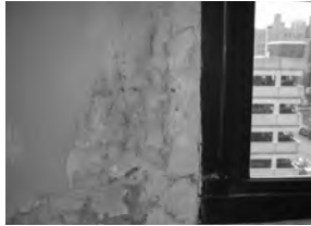
Interior finish damage.
