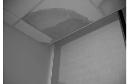
Water intrusion and interior damage.
