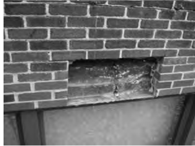
Damaged flashing at window head.
