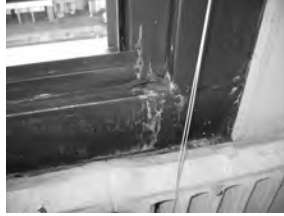
Stains on frame.
