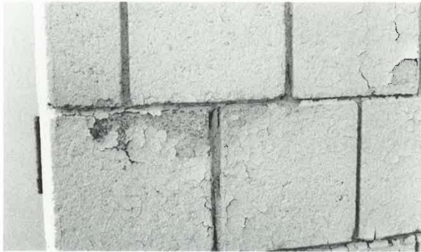
Coating is peeling as a result of water trapped within the masonry wall.
