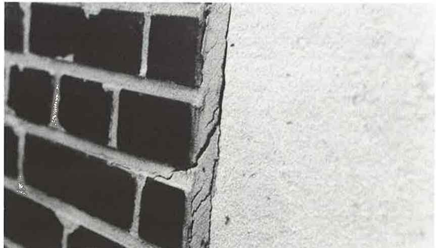
Cracks in the masonry mortar
