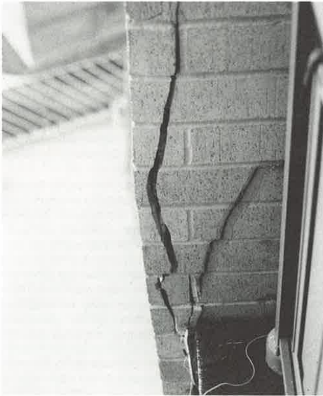
Vertical displacement of brick veneer
