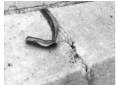
▲ Lead joint cover has been pushed out of the joint. Caulking in joint is brittle and not bonded to the stone.
