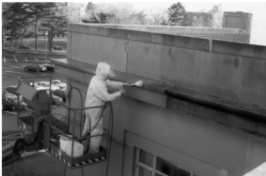
▼ (Below) A worker scrubs and removes softened soil from the water-soaked limestone façade.
