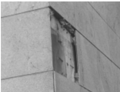
Damaged stone has been removed, exposing the concrete back-up wall.
