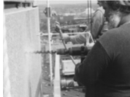
Step 1: Drilling the stone and back-up wall in preparation for the anchor.
