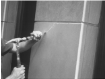
A worker removes failed patching material from a crack in the limestone facade.
