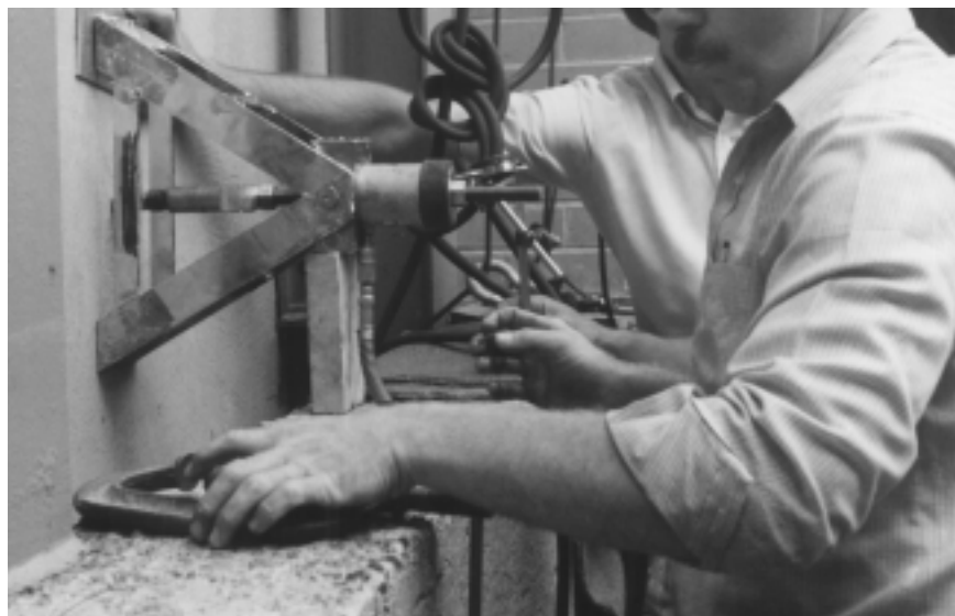
A pull-test in the back-up wall is used to evaluate anchorage performance.
