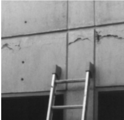
Severe spandrel spall over east entrance of Xerox Document University.
