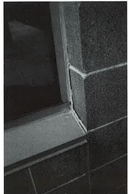
An example of adhesive failure between the sealant and the concrete block and between the sealant and the painted metal window edge.
