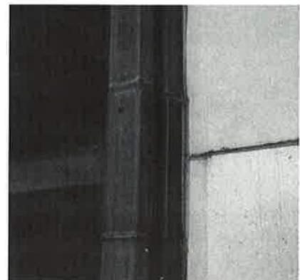
Poor joint design has placed dissimilar materials together; differing expansion/contraction rates increase stress on the sealant joint, leading to sealant failure.
