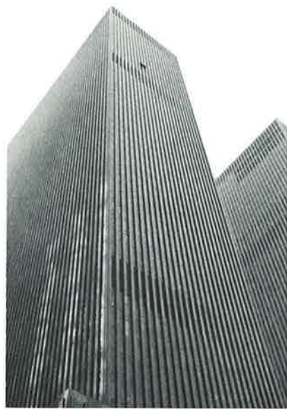
The swing staging high on this building carries a work crew performing remedial sealant work specified and monitored by Hoffmann Architects.
