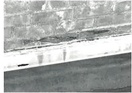
Missing weep holes.
