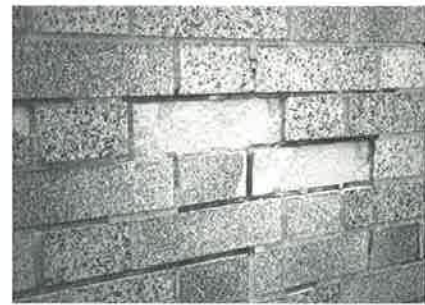
Spalling of glazed brick.
