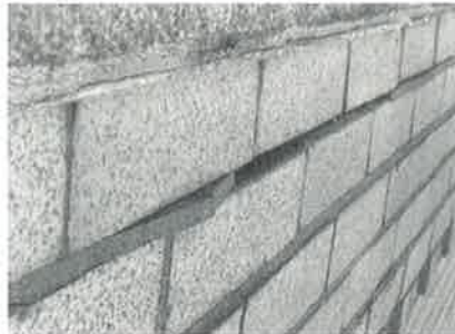
Deterioration and missing mortar at joints.
