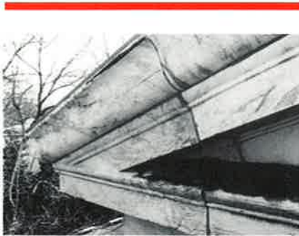
Pediment detail shows effects of stone displacement.
