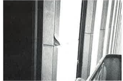
Spalling at joint between limestone panels.
