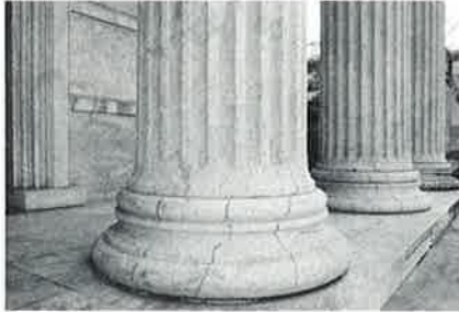
Severe cracking at base of marble column.
