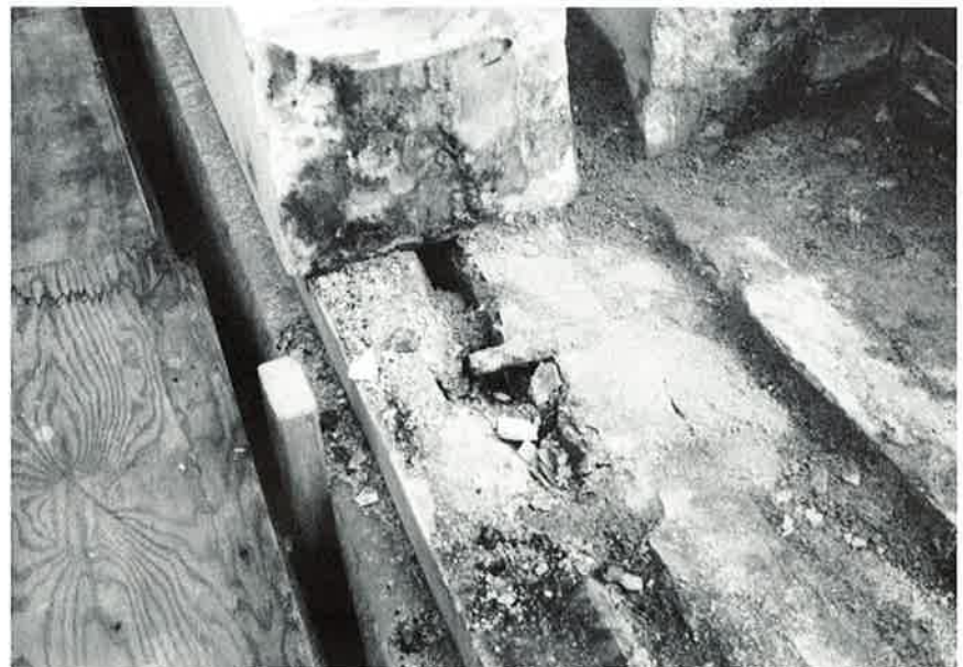
Stone has been removed to examine metal anchor, which has corroded and broken.
