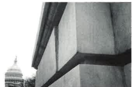
Water infiltration has caused stone section to shift from original position.
