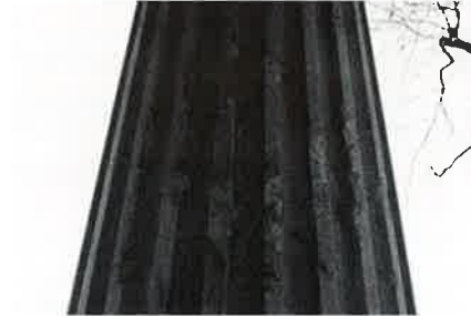
Heavy spalling and exfoliation on column shaft.
