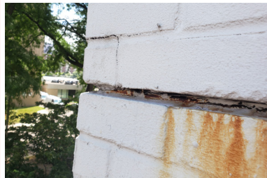
▲ Rusted relieving angle and failed sealant.
