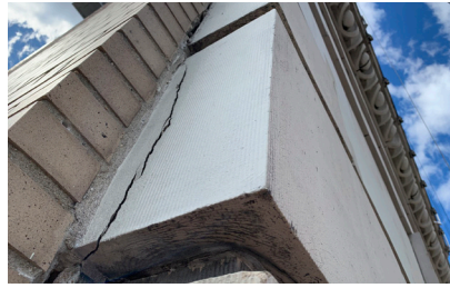
▲ Unsafe conditions pose immediate danger.
