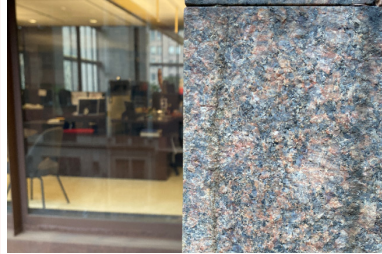
▲ Hairline cracks in granite.
