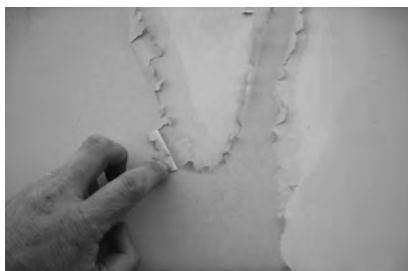
A Peeling coatings
