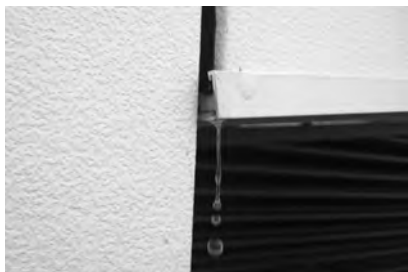
A Movement and water intrusion
