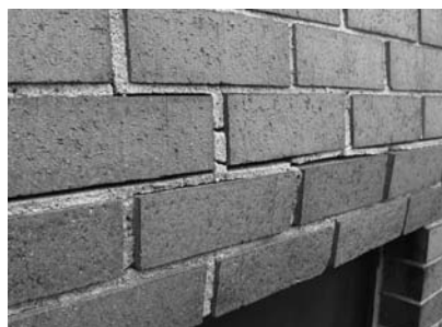
▲ Bowing and displacement in brick masonry are symptoms of restrained movement.
