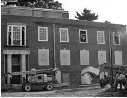
▲ The challenge is to select windows that suit the building and perform as desired.
