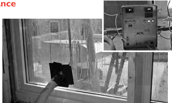
▲ On-site air and water leakage testing can provide a quantitative measure of in-situ window performance.
