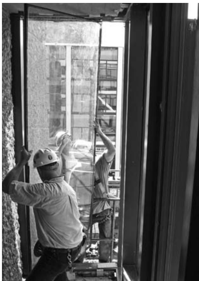
▲ Insulating glazing may be heavier than the original glass, requiring additional support.
