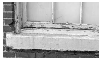
▲ Wood window coating deterioration.
