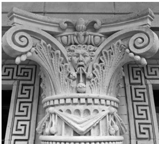
▲ The coating on this decorative terra cotta element protects the surface from exposure.
