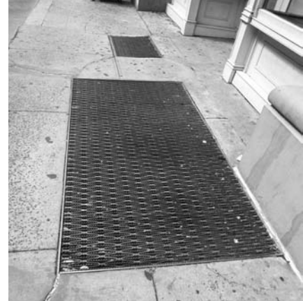
▲ Falling into a faulty grate is a real concern.
