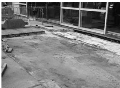
▲ First, the concrete wearing surface is removed to expose the concrete vault.
