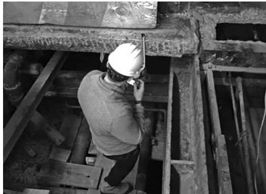
A An engineer investigates structural slab conditions at a partially deconstructed sidewalk vault.
