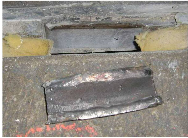
Figure 5 Fatigue failure of flat bar-type connection.
