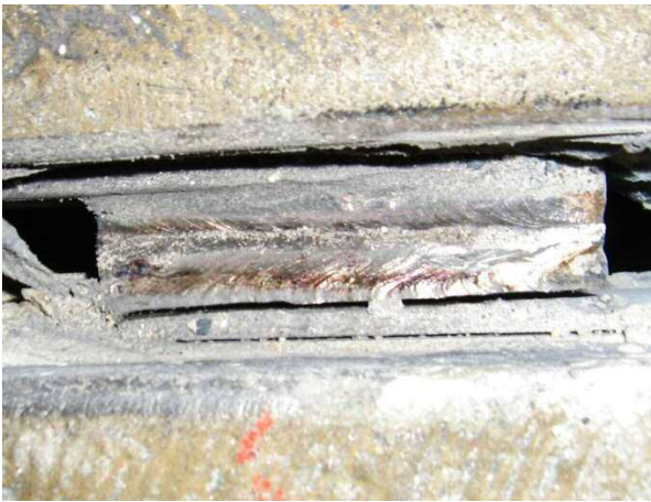
Figure 6 Fatigue failure of flat bar-type connection.
