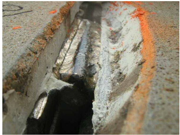
Figure 7 Fatigue failure of dowel-type connection.
