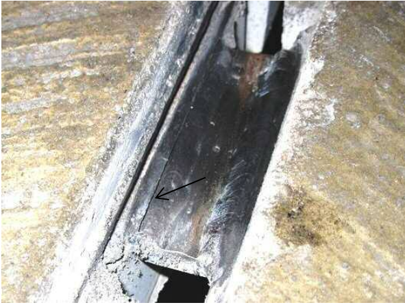
Figure 4 Fatigue failure of flat bar-type connection.
