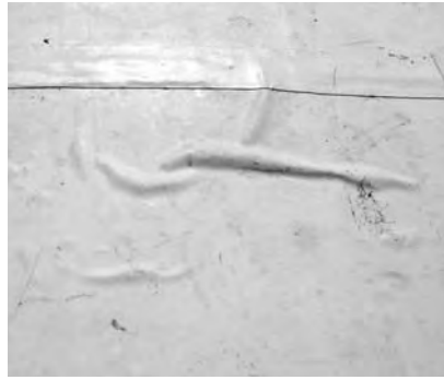
A Blisters and wrinkles are common problems for sheet membrane assemblies.
