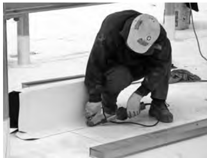
▲ Edge detailing is just as important on a cool roof as on a conventional one.
