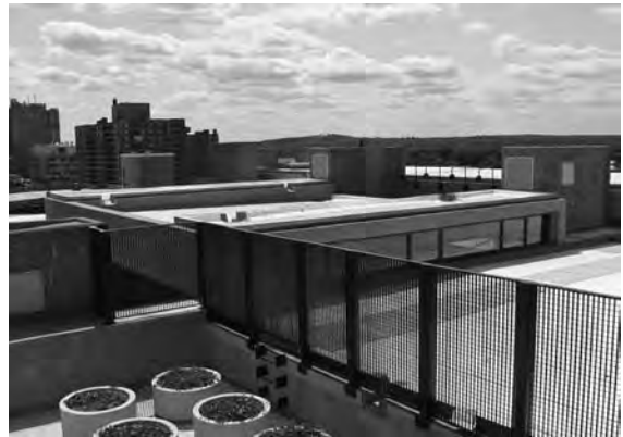
▲ Yale University, Paul Rudolph Hall (Art + Architecture Building) in New Haven, Connecticut. Roof Replacement and New Construction Consultation – Vegetative Roof and Cold-Applied MBR System with Reflective Cap Sheet.
