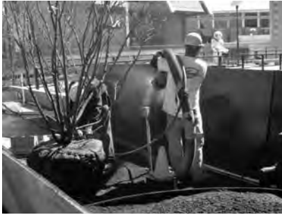
A Installation of planting medium around a large shrub on an intensive green roof.
