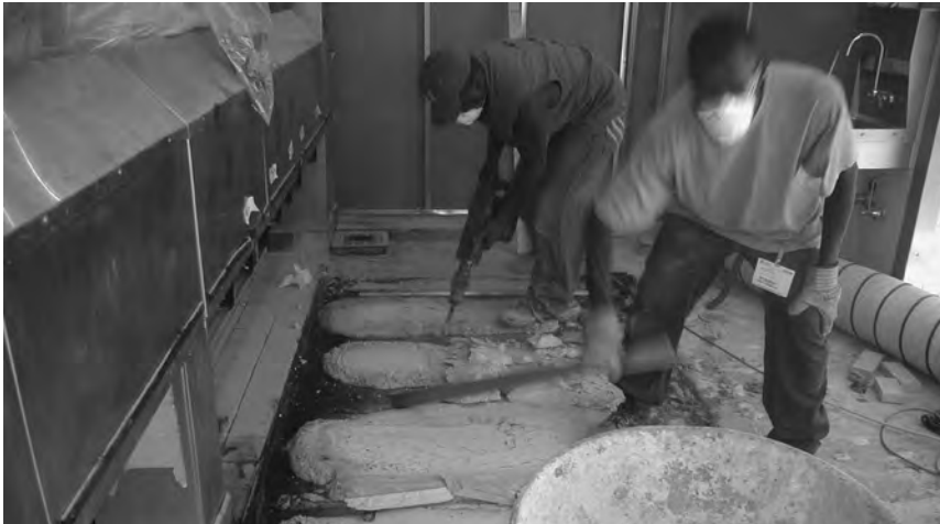
▲ Suspending kitchen operation for waterproofing rehabilitation is hardly desirable. But if leaks are ignored, water damage to structural systems and finishes will only make things worse.
