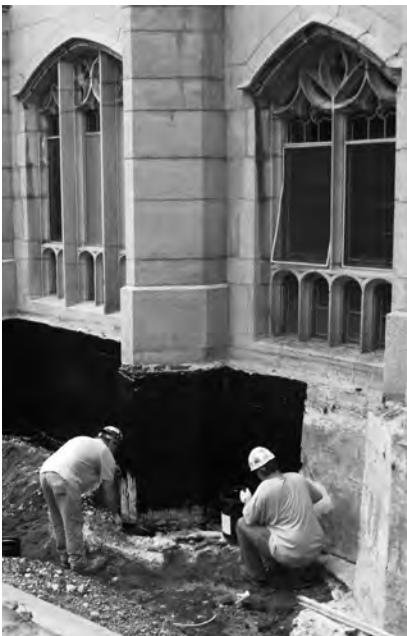
▲ Once below-grade waterproofing is buried, leaks due to faulty application can be difficult to resolve.
