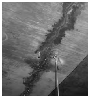
▲ Leaks at underside of deck.
