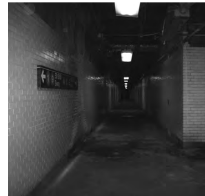
▲ Pedestrian tunnels offer convenient access, but their location under busy areas makes waterproofing particularly challenging.
