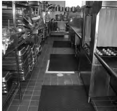
▲ Dishwashers and other kitchen equipment introduce a high-volume water source with a high potential for leaks.
