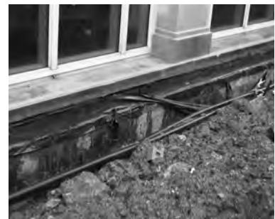
▲ Positive side waterproofing defects, viewed during repair excavation.
