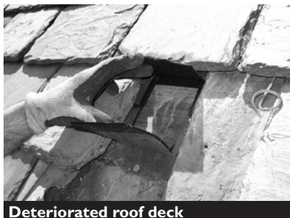
Deteriorated roof deck
