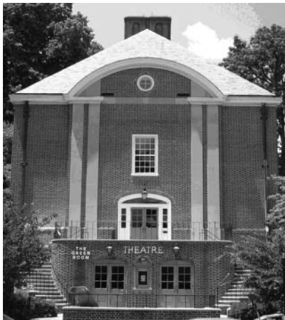
▲ Keiper Hall/Green Room Theater (1936) at Franklin & Marshall College in Lancaster, PA. Masonry Restoration.
