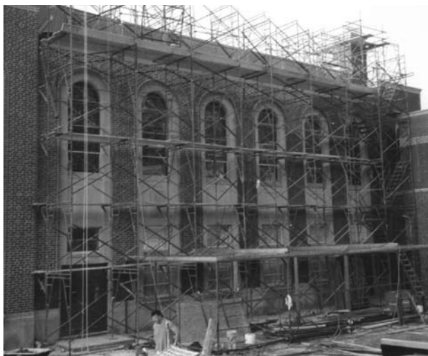
▲ Thoughtful organization of repair work will minimize disruption and costs associated with erecting scaffolding and construction equipment.
