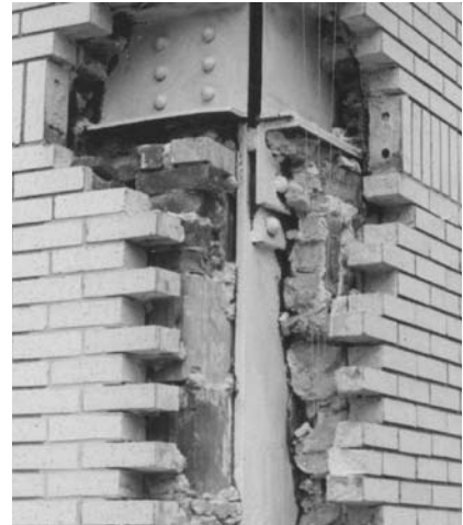
▲ Addressing the root causes of masonry distress avoids wasting time and money on duplicate repairs. Here, replacing rusting steel supports before rebuilding the face brick provides a long-lasting solution.
