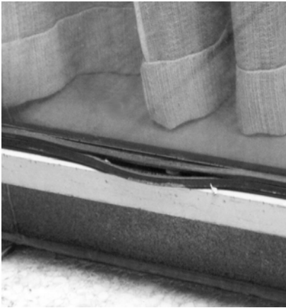
A Figure 3. Failed gasket at the base of the glazed curtain wall will permit water and air penetration.
