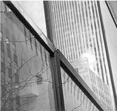
A Figure 4. The metal support system behind the mullion cover has rusted, causing it to extrude.
