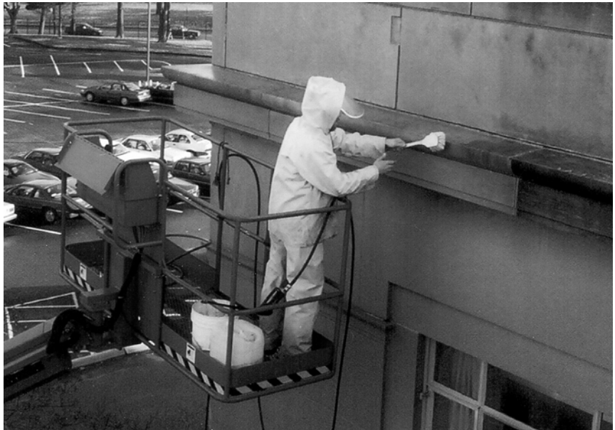
A worker scrubs and removes softened soil from the water-soaked limestone façade.
