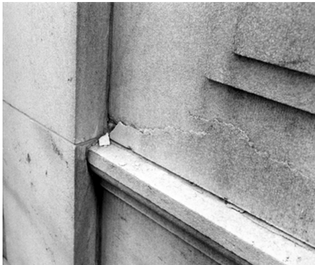
A Large spall is shown in limestone panel above window
