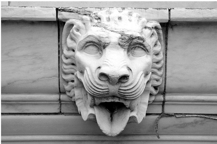
A Inappropriately applied sealant is failing, or missing altogether, in joints. Areas of the sculpture are beginning to show signs of erosion.
