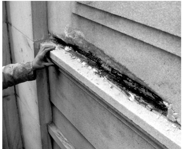
A Removal of spall exposes corroded steel beam behind stone panel.
