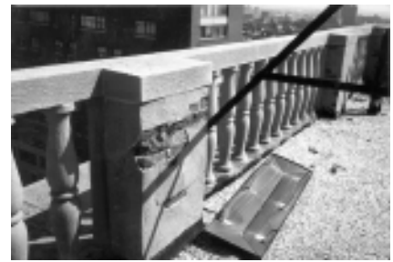
▲ In this case, a cementitious coating left the brick parapet saturated with trapped moisture, which eventually caused spalling and crumbling of the masonry.
