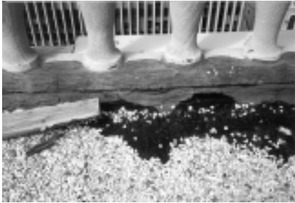
▲ Inappropriate repair measures can do more harm than good. Here, roofing mastic used to patch this balustrade base led to further water retention and deterioration.
