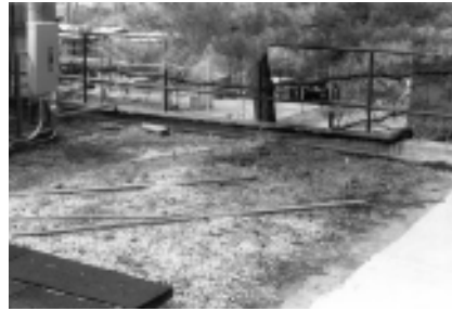
▲ While attractive as landscaping elements, trees can pose problems when allowed to overhang a flat roof for an extended period of time. This tree's shed pinecones and needles retain moisture and provide an ideal climate for bird nesting and organic growth, both of which can severely damage roofing materials.
