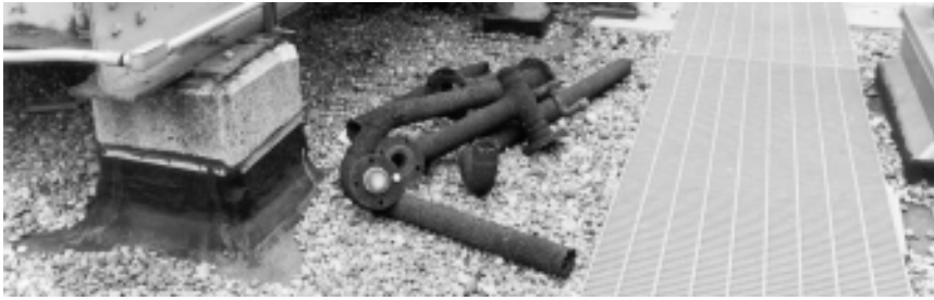
▲ Mechanical debris lies directly on the roof membrane. Not only may this lead to deterioration, but it may also prevent the safe inspection of the roof.
