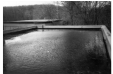
▲ A dramatic example of ponding , or water retention on the roof membrane.
