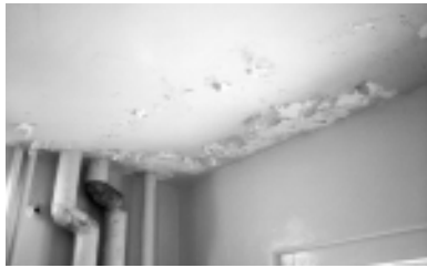
▲ One of the most noticeable and, often, most troublesome signs of a failed roofing system is interior water damage.
