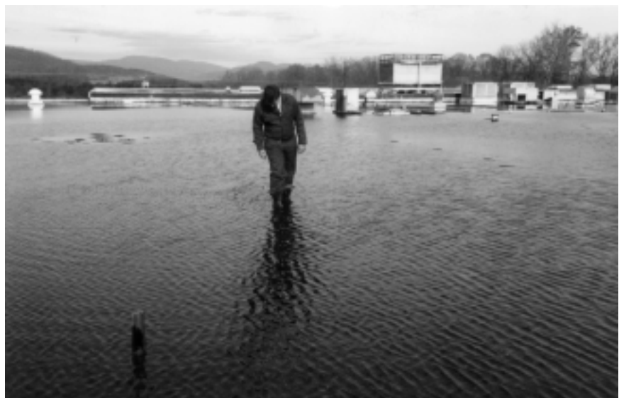
The ponded water on this roof could add enough weight to cause collapse.
