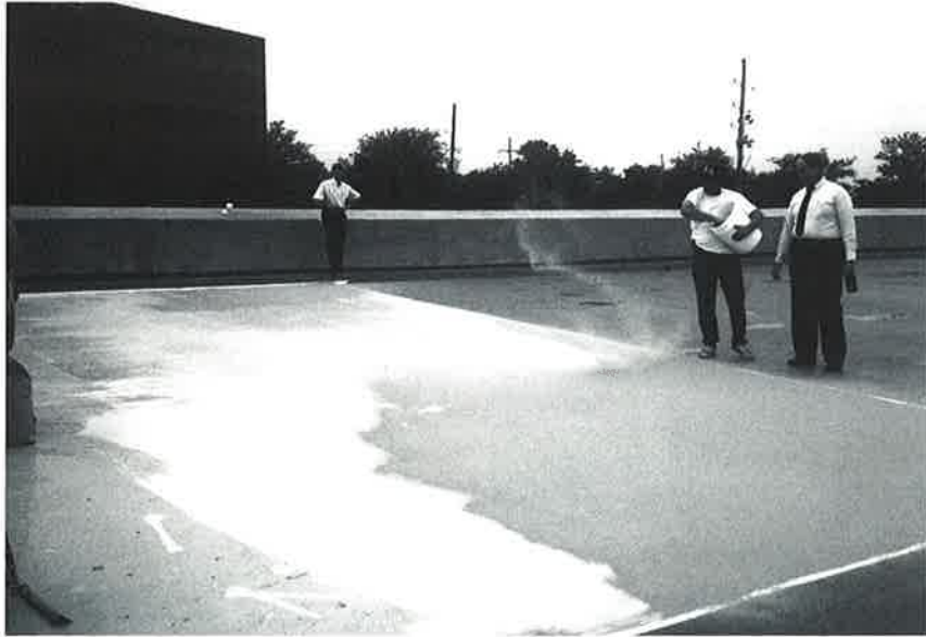
The aggregate is applied to provide a skid-resistant surface and is then covered with the top coat; together, these make up the wear surface.
