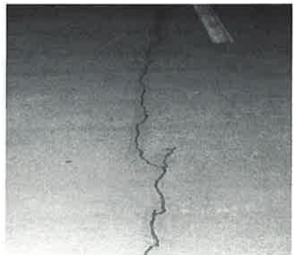
Large cracks, such as that shown above, must be routed and sealed before the detail and base coats are installed.
