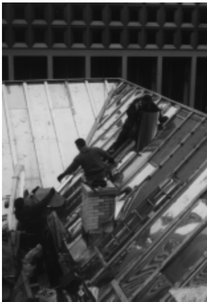
Installation of a batten seam copper roof on a New York City high-rise office building.
