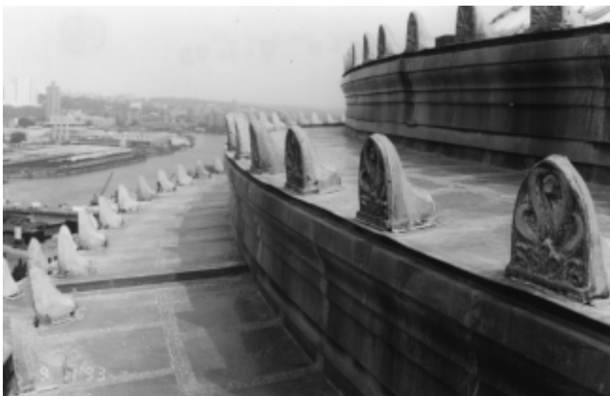
A previous attempt to solder over these failed flat seam joints was not successful.
