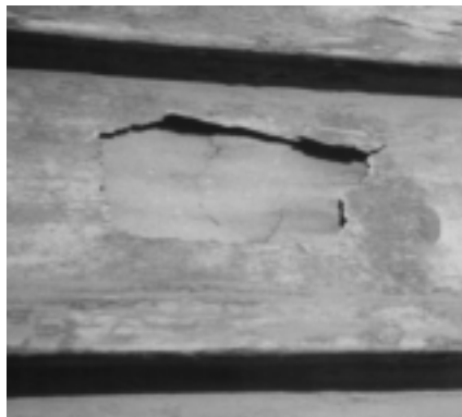
This copper roof failed — after 70 years of service and acid rain.
