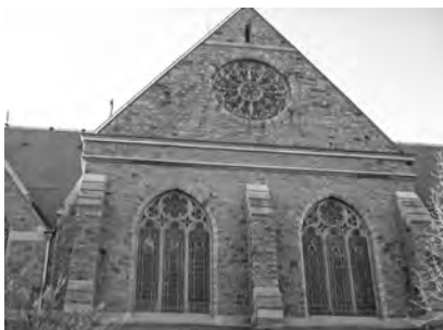
▲ Packer Memorial Church (1885), Lehigh Univ., Bethlehem, Penn., Masonry Restoration and Window Replacement/Rehabilitation.
