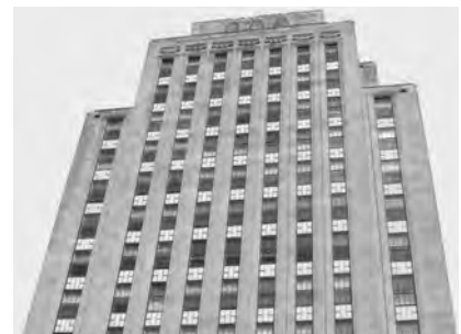
▲ Former Southern New England Telephone Headquarters (1938), New Haven, Conn., Steel Window Refurbishment.
