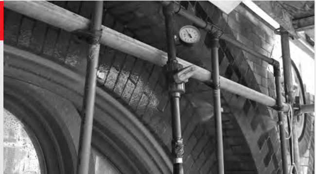
▲ In the field: Spray rack water test of a rehabilitated historic window.
