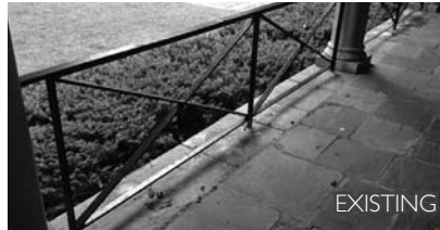
▲ Railings at historic terrace are too low, with openings that are too large.
