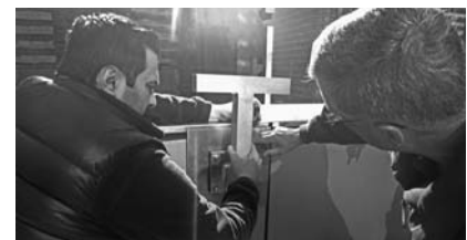
▲ Thicker insulation due to new energy code raises roof surface and demands taller railings.
