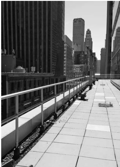
▲ As codes change, owners may find that existing railings must be updated or replaced.
