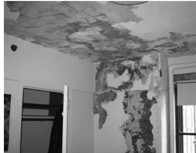
▲ Interior finish damage from roof leaks.
