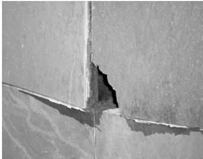
▲ Displacement and fracture at stone facade.
