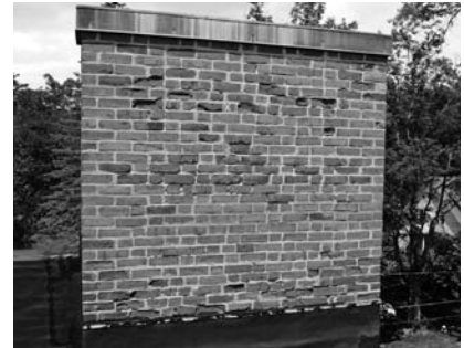
▲ Spalled brick masonry at chimney.
