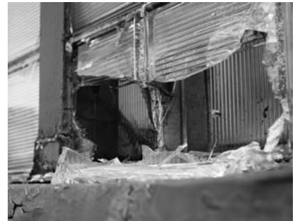
▲ Shattered glass block windows.
