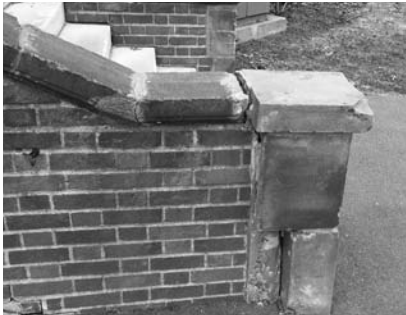
▲ Site wall and exterior stair damage.
