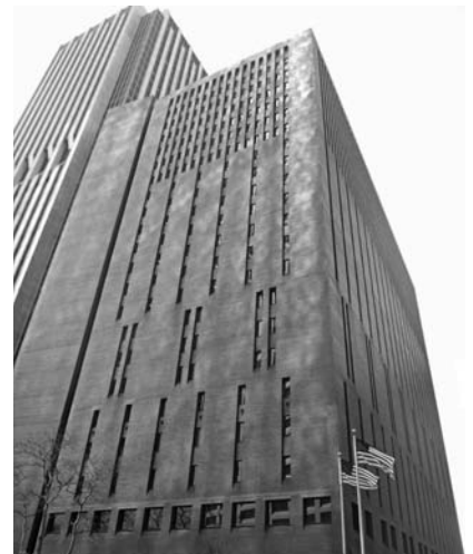
▲ Edge Fund Advisors, 4 New York Plaza in New York, New York. Facade Investigation and Rehabilitation.
