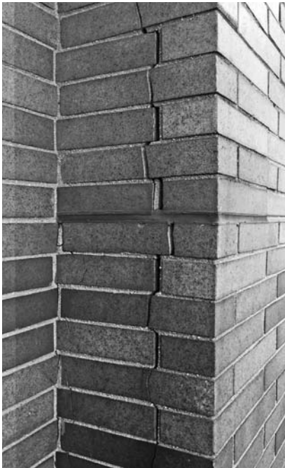
▲ Long, vertical cracks at building corners may indicate underlying structural distress.
