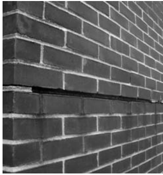
▲ Corrosion of steel shelf angle.
