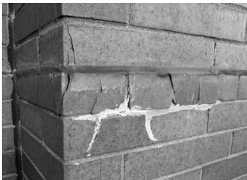
▲ Sealant alone cannot resolve masonry distress.
