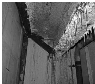
▲ Figure 3b: Plaza leaks corroded steel and melted fireproofing beneath the faulty joint.
