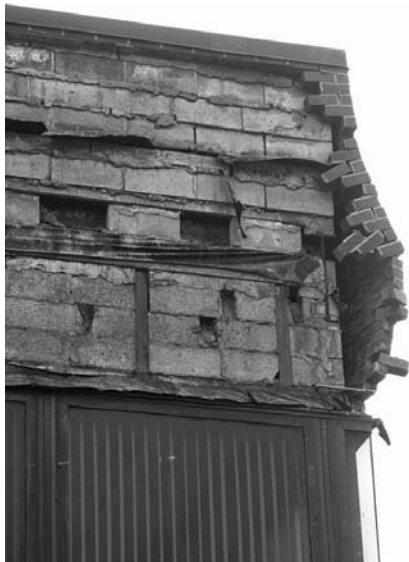
▲ Unless the problem is correctly diagnosed and repaired, it will continue to worsen, sometimes to the point of major failure.
