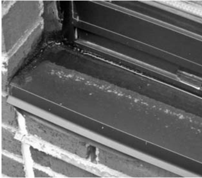
▲ Figure 1a: Masonry expansion led this sill to bend upward at the front edge.
