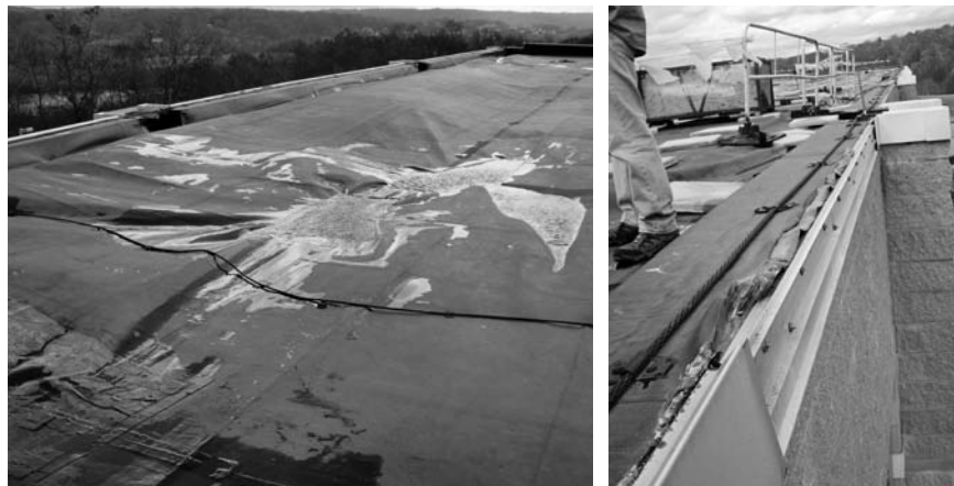
▲ Figures 6a (left) and 6b (right): Roof blow-off caused by insufficient insulation adhesion, poor edge detailing, and other construction defects.
