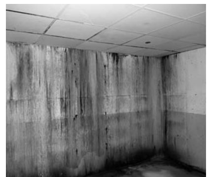
▲ Figure 3c: The plaza looked great, but leaks left rooms below looking anything but.
