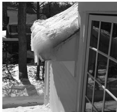
▲ Figures 7a (top) and 7b (bottom): Ice dams at eaves led to extensive leaks at the building interior and required replacement of the roof just a few years after it was installed.
