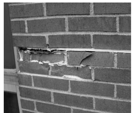
▲ Figure 2b: An attempt to fix spalled brick with sealant made matters worse.
