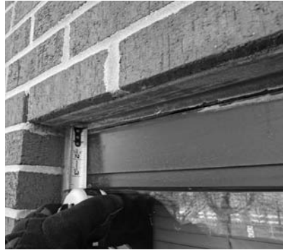
▲ Figure 1b: As the brick veneer expanded, it pulled upward away from the window.
