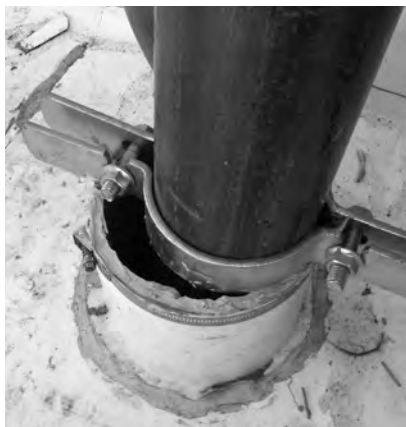
A An open pipe penetration spotted during a waterproofing consultation.
