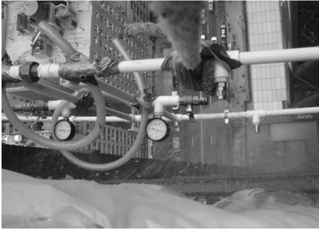
▲ High-rise buildings pose logistical challenges to water testing, including securing the test apparatus and managing overspray.
