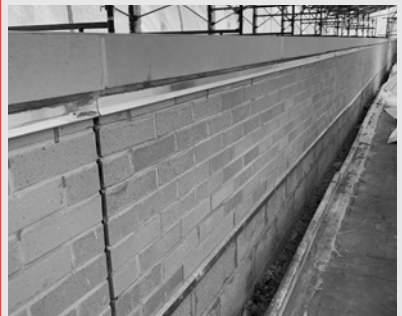
▲ With the copings and flashing in place, the parapet is nearly complete.
