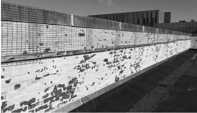
▲ Unstable parapets may be secured temporarily with netting.
