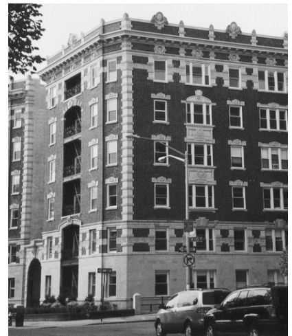
▲ Columbia University, 44 Morningside Dr., New York, NY, Building Envelope and Parapet Rehabilitation.
