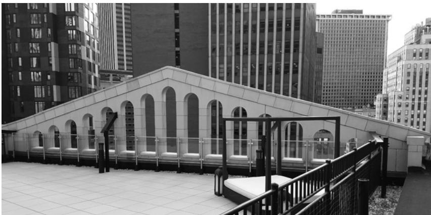
▲ Parapets vary from plain to ornate, but all must provide stability and moisture protection.
