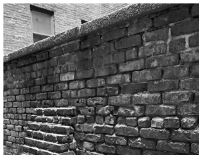
A Open mortar joints lead to deterioration.
