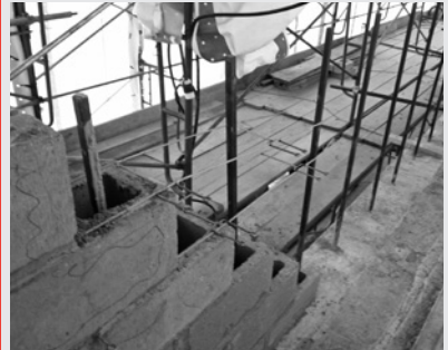
▲ Steel bars reinforce the concrete masonry unit core of the new parapet.
